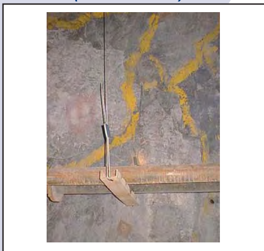
Pipe Rack - Underground Mine
